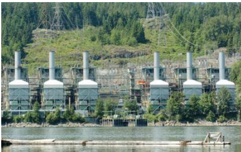
Burrard Thermal power plant in Port Moody burns natural gas to generate electricity.
